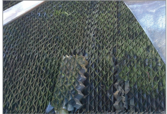
Figure 5.4-3: Damaged drift eliminator sections with algal build up
