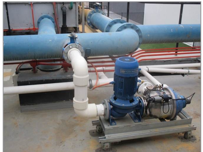
Figure 5.1-3: Side stream filtration equipment at the balance line, connecting three cooling tower basins
