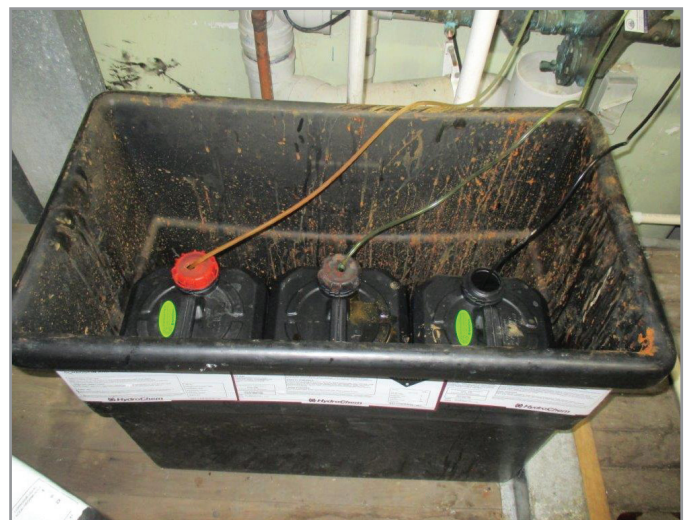
Figure 5.3-5: A bund container that may compress dosing tubes when the lid is replaced
