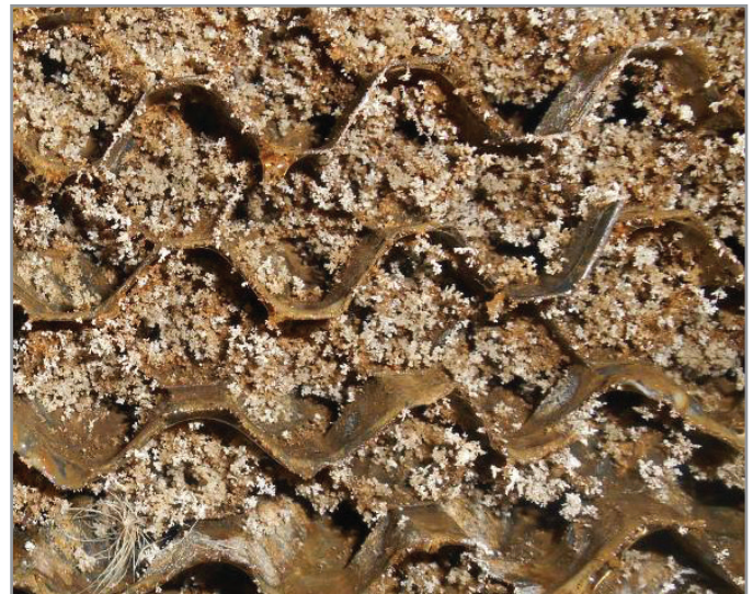
Figure 5.3-2: Significant scale build up in the fill material
