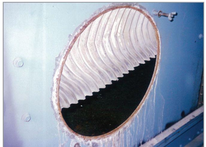
Figure 5.4-2: Collapsed fill can affect thermal performance and block access for maintenance
