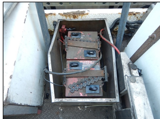
Image 4 – Damaged enclosure on back of utility
