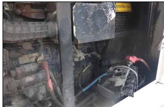
Image 2: Failed battery in 100kVA generator
