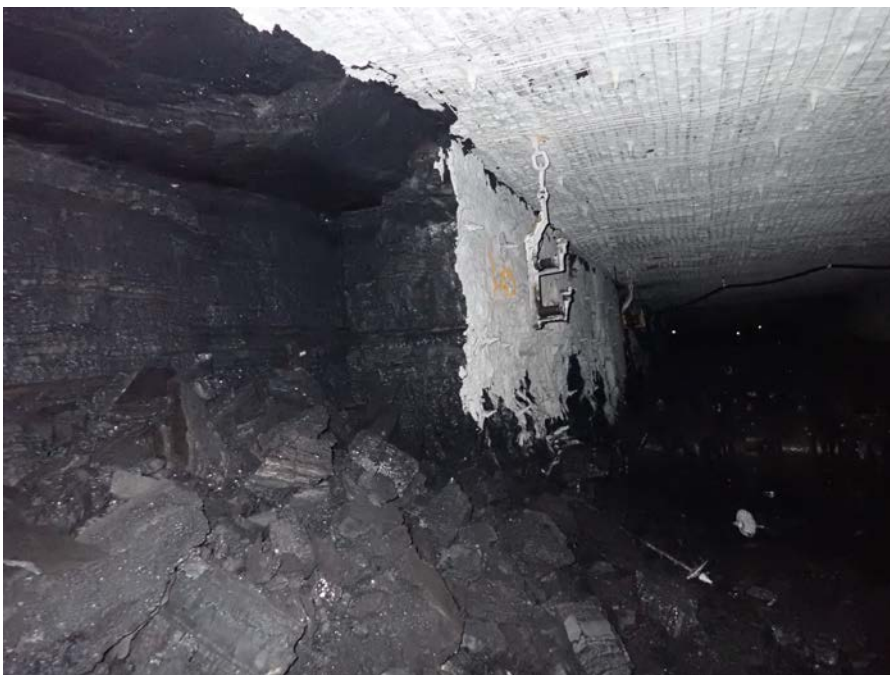
Figure 3 – Failed section of rib (SinNot-2018/00638).
