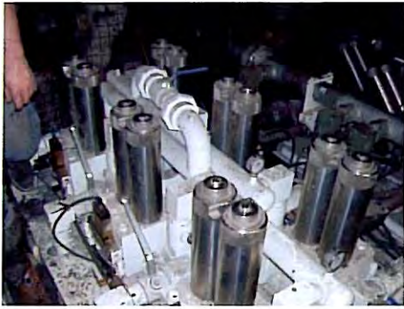
Longwall filter station
