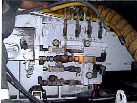
Stagel loader discharge flow meter panel
