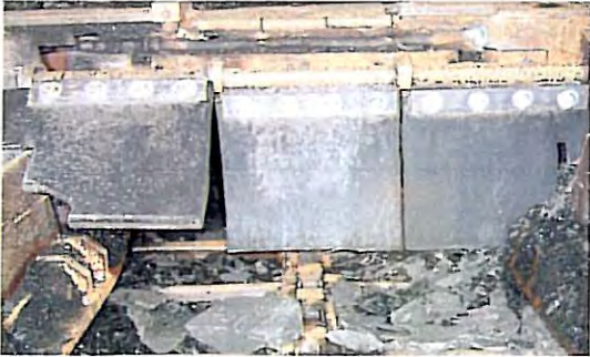
Conveyor belt door
