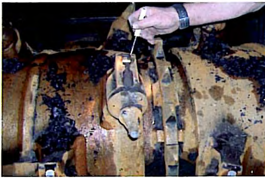
Wet head spray location
