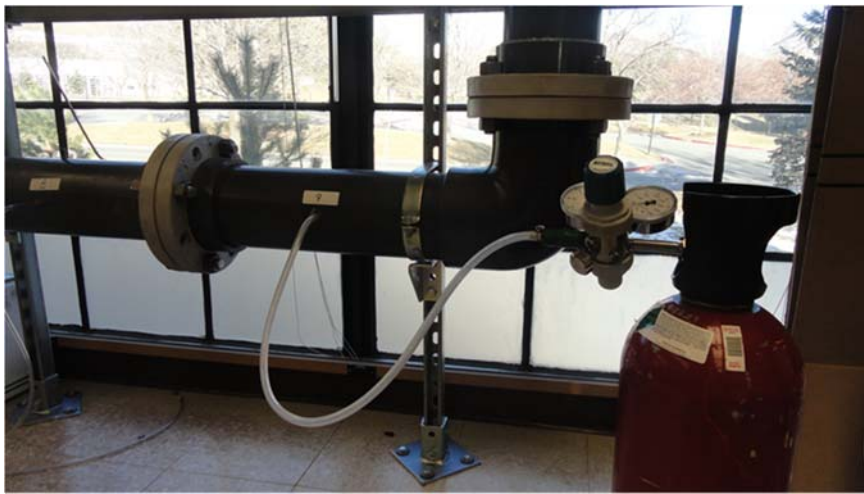
Figure 5.5. CO 2 Gas injection system
