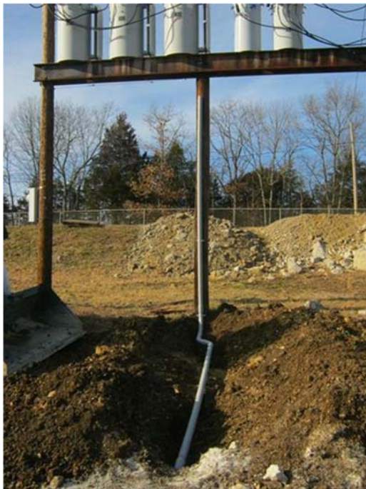
Figure 6.4. A 76-mm drill hole with the 50-mm conduit passing wire to underground
