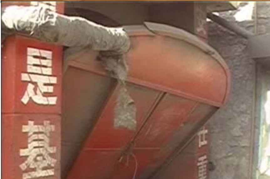
A destroyed air door near a shaft
