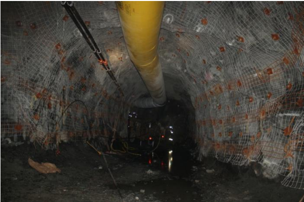
Uncontrolled Ground Movement
