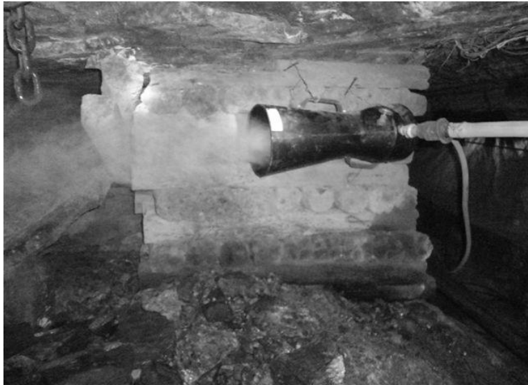
Figure 5: One of the underground installations at the trial site at Beatrix Gold Mine
