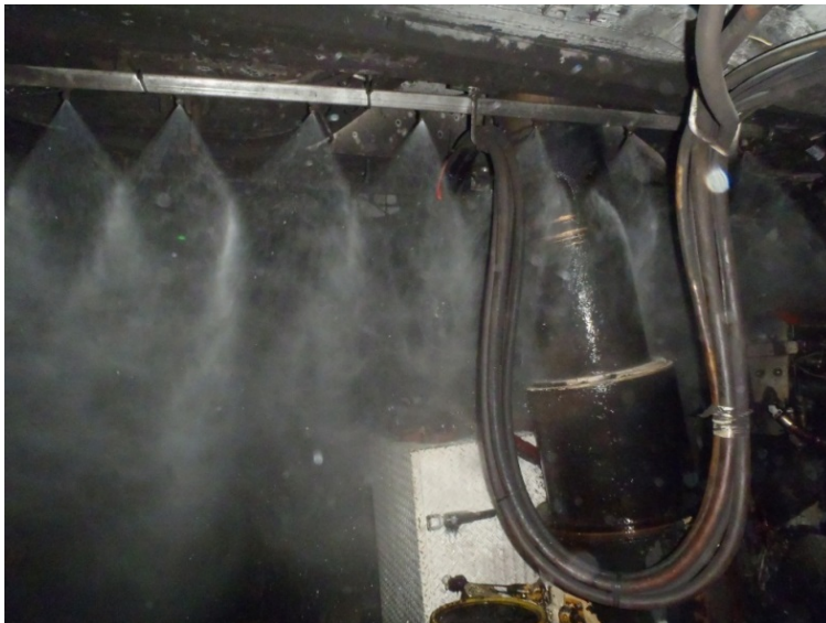
Figure 9: Face partition sprays installed on a shield canopy
