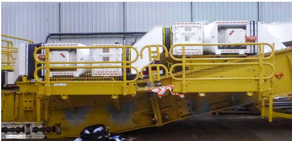
Figure 2: Scrubber fan system mounted on BSL
