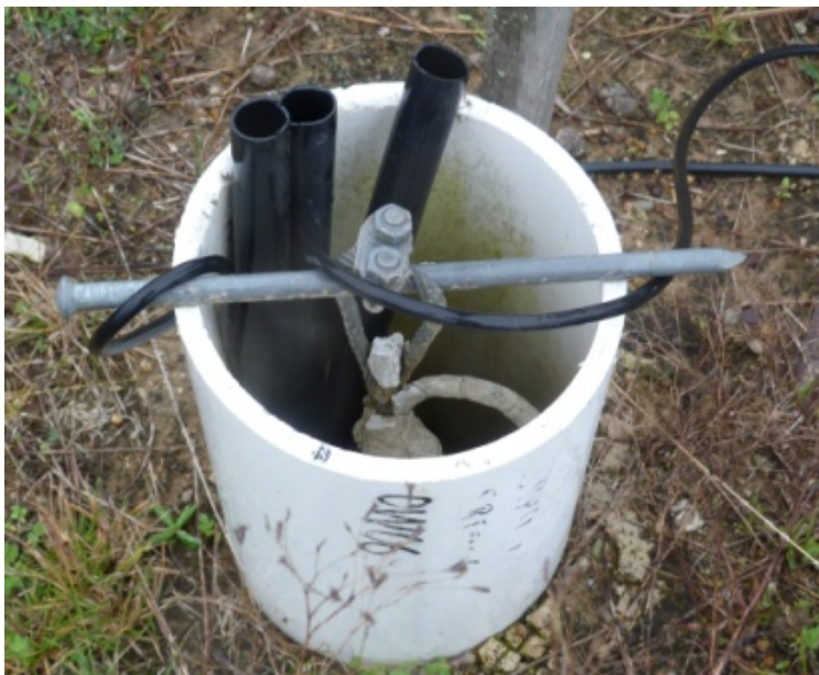
Figure 29 - Photo looking at the top of typical piezometer hole at Blakefield South Mine.
