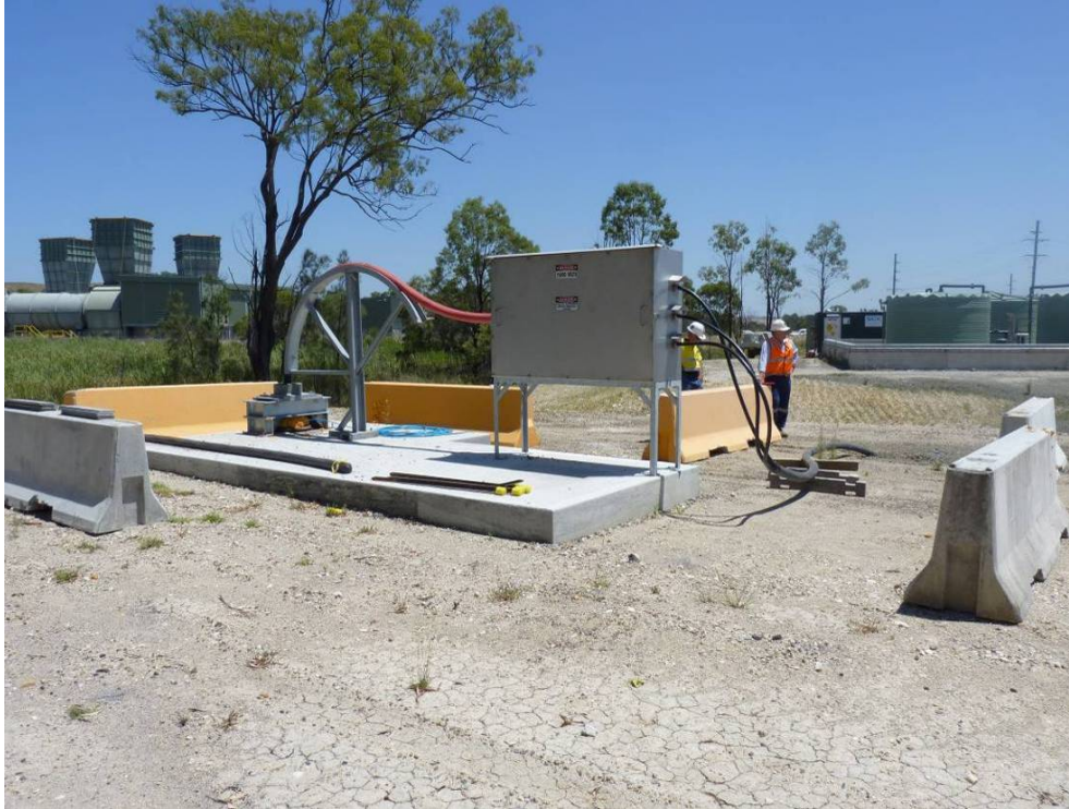
Figure 26: Junction box and entry point for LW1 11 kV cable entering Blakefield South Mine. Note: the installation is not fenced and cable leading into the junction box is unprotected.
