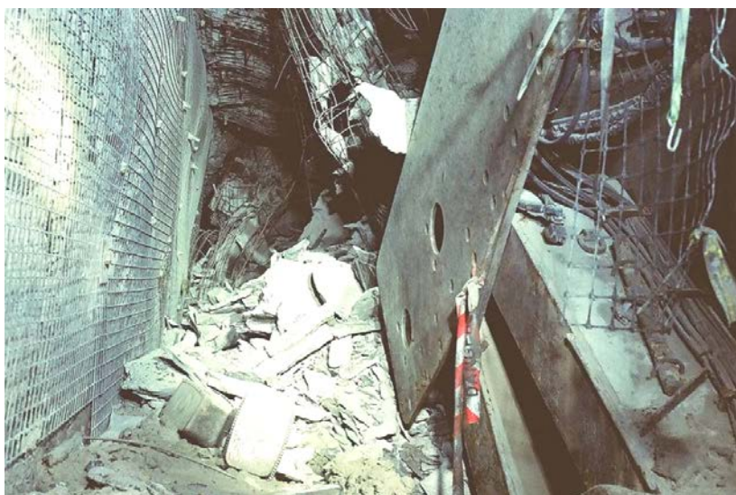
Figure 19: Looking at the goaf between the chain pillar rib and chock 1 at the main gate
