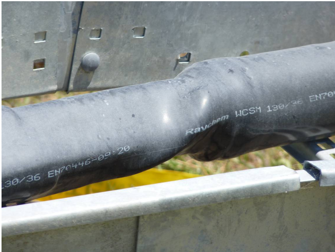
Figure 28 – High tension cable joint showing poor quality join
