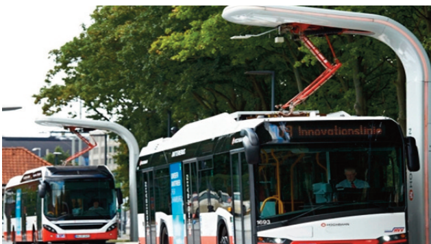
Figure 7. Pantograph Overhead E-Bus Charger (Siemens, 2017)
