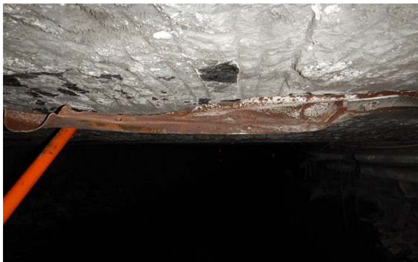
Figure 14: Remaining section of W strap that was involved in incident showing signs of previous impacts.
