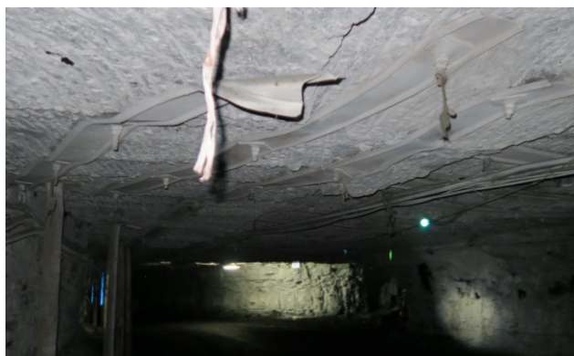
Figure 12: Damaged W straps the vicinity of the incident.
