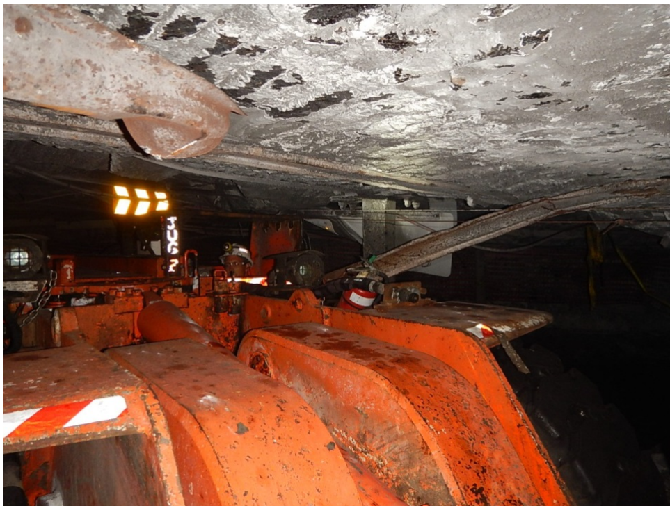
Figure 7: Position of W strap and similar type of machine - looking outbye toward the scene.
