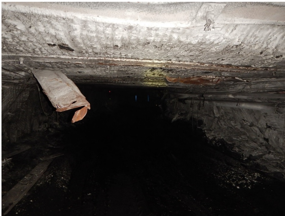
Figure 5: Damaged W strap hanging in roadway looking inbye at the scene
